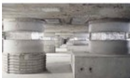
IoT and Cloud Support Center operated in a dedicated facility complete with earthquake resistance and backup power supply
